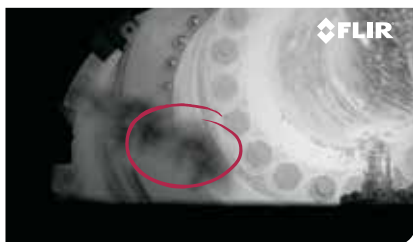
A leaking flange.
